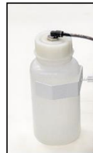
Fig. 16: Check of condensate collection vessel
